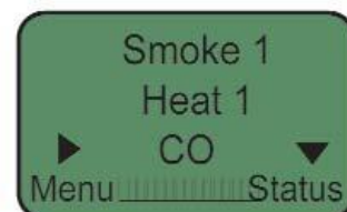
Example of a simultaneous testing (smoke + heat at the same time)
